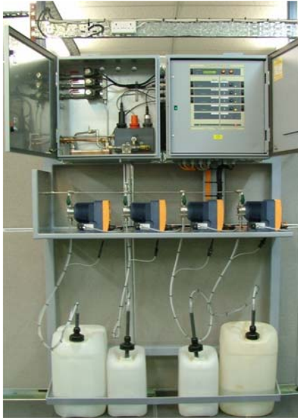
AQ300LP System for feed and 2 boiler samples (up to 10 bar) with 4 chemical dosing pumps controlling oxygen scavenger, condensate treatment and a boiler product to each boiler., this unit also controls blowdown
