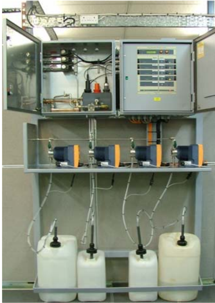
AQ300 System for Feed and 2 boiler samples controlling 4 chemical dosing pumps: Pump for Oxygen Scavenger Pump for Condensate conditioner Pump for Boiler Product for each boiler
